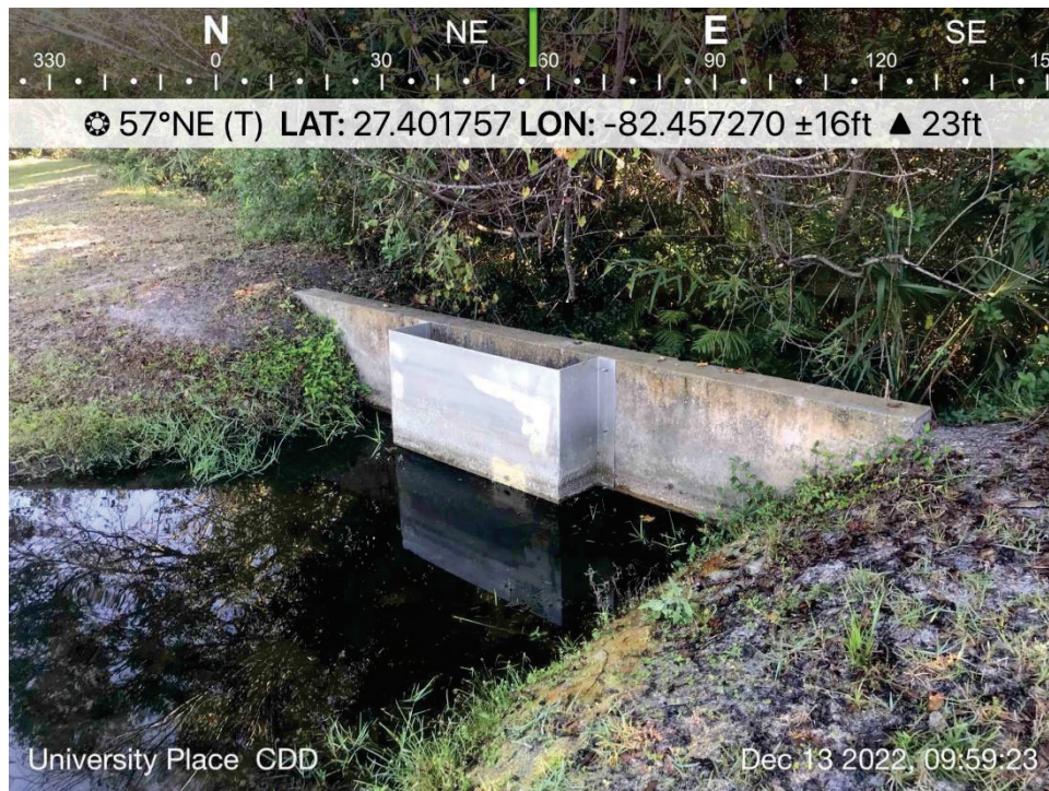
POND 1 – View of CS #UP1A. Operating normally, low water levels, monitor wing wall ends for minor erosion.
