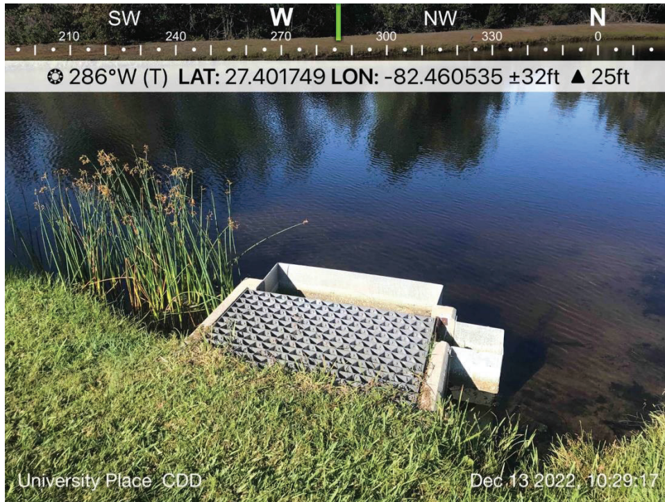
POND 3 – View of CS #UP3, Operating normally, low water level, monitor potential erosion on north side. Recommend removing metal grate in weir.
