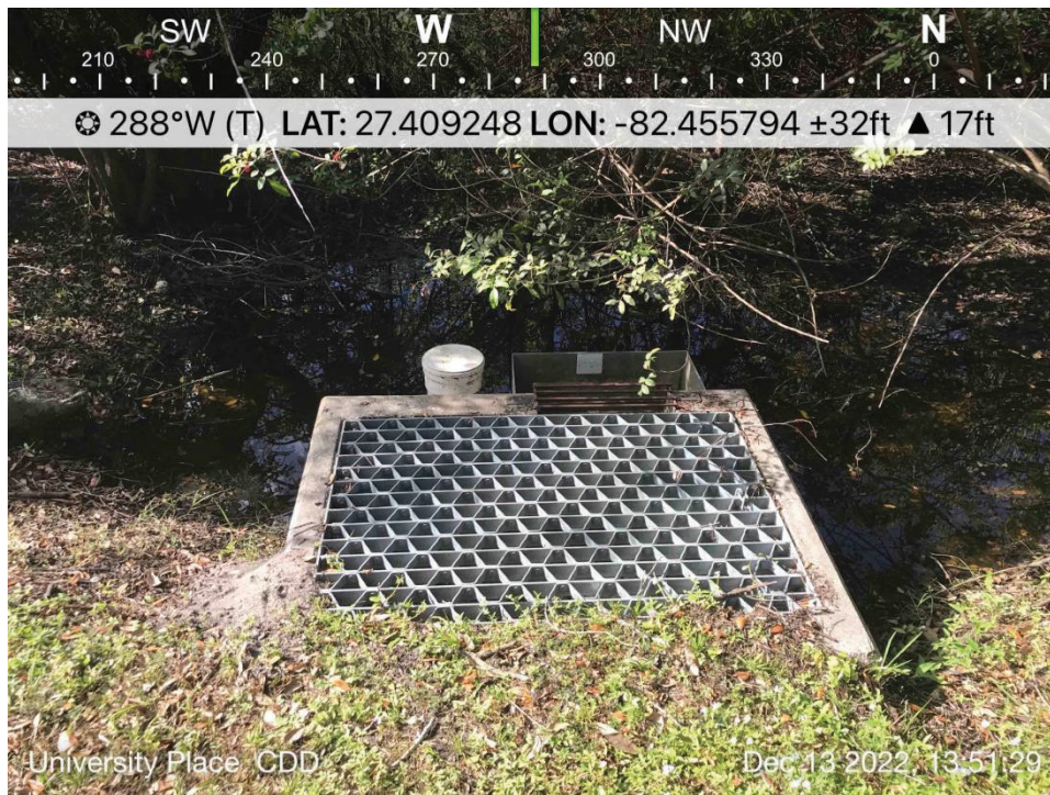
POND 14 – View of CS #UP14. Operating normally, low water levels, recommend removing metal grate at weir.
