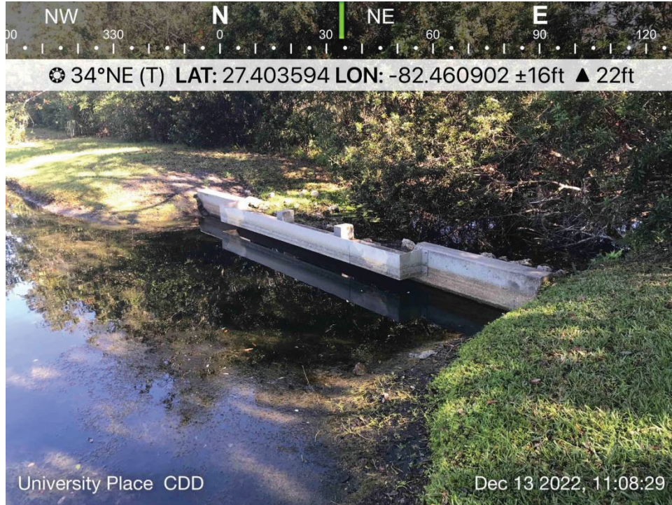
POND 6 - View of CS #UP6. Operating normally, low water levels, recommend future repair for wing wall end erosion.
