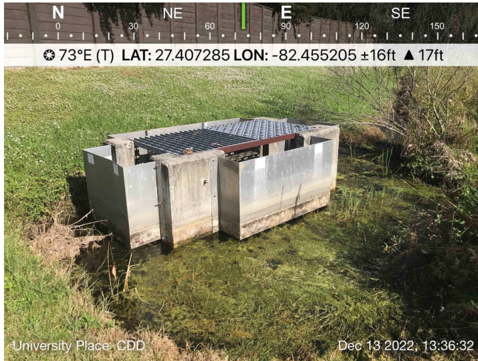
POND 13 – View of CS #UP13. Operating normally, low water levels.
