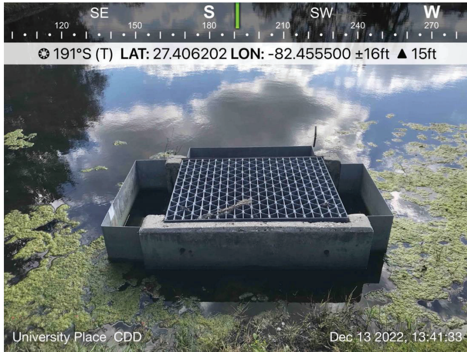
POND 15 – View of CS #UP15. Operating normally, low water levels.
