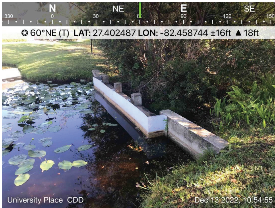
POND 5 - View of CS #UP5. Operating normally, low water levels, monitor wing wall ends for minor erosion.
