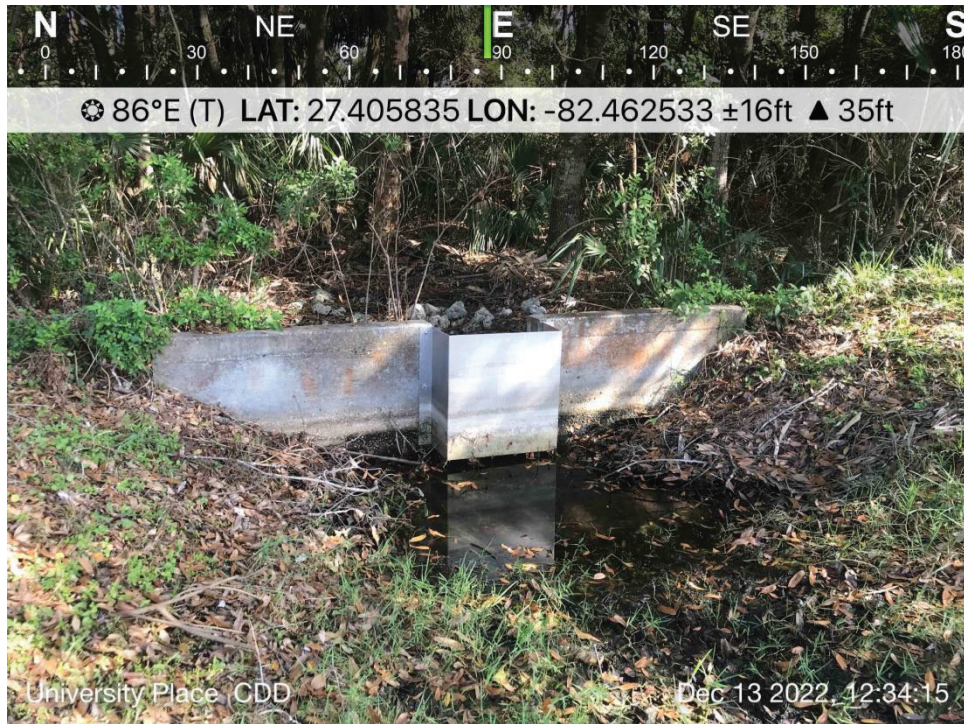
POND 8 - View of CS #UP8. Operating normally, low water levels.
