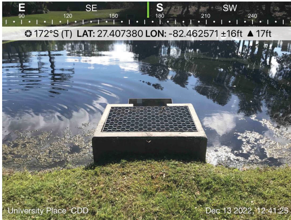
POND 9 – View of North CS #UP9-J. Operating normally, low water levels.
