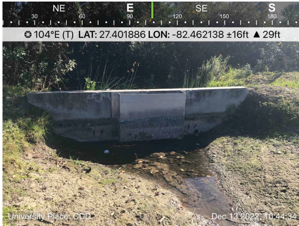
POND 4 - View of CS #UP4. Operating normally, low water levels, monitor wing wall ends for minor erosion.
