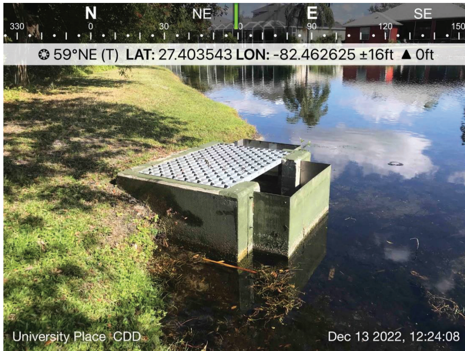
POND 7 - View of CS #UP7. Operating normally, low water levels.
