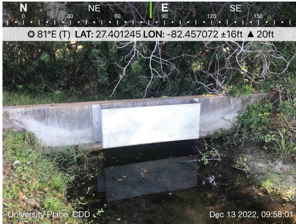
POND 1 – View of CS #UP1B Operating normally, low water levels, recommend removing vegetation from around CS.
