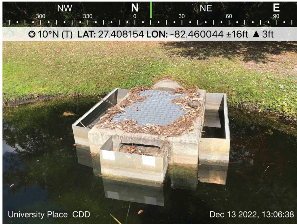
POND 11 – View of CS #UP11. Operating normally, low water levels, recommend removing debris from structure.
