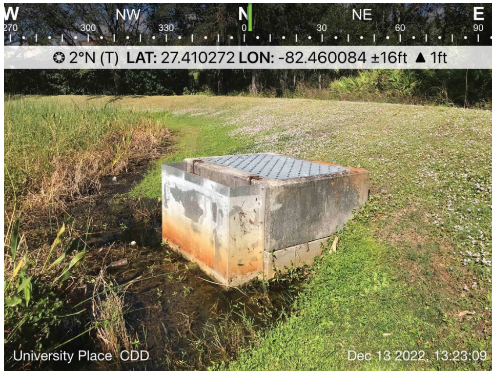
POND 12 – View of CS #UP12. Operating normally, low water levels, recommend removing metal grate at weir.
